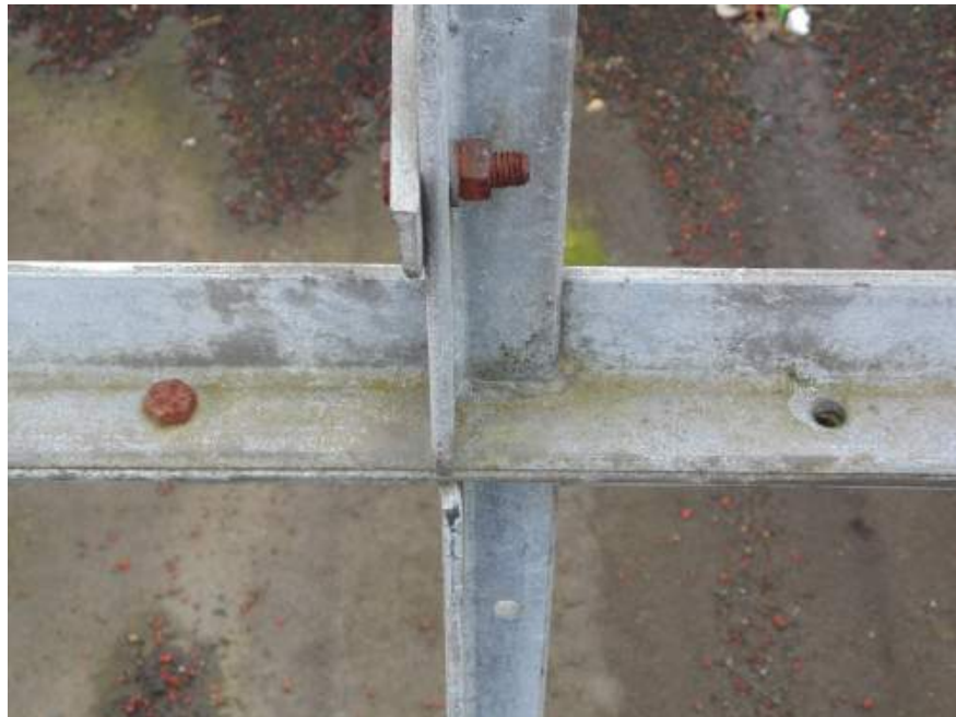
FIGURE B6: RUSTED SCREWS
