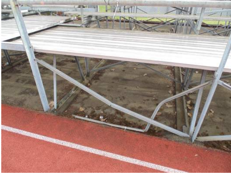
FIGURE S6: DESTROYED CROSS BRACE ANGLE
