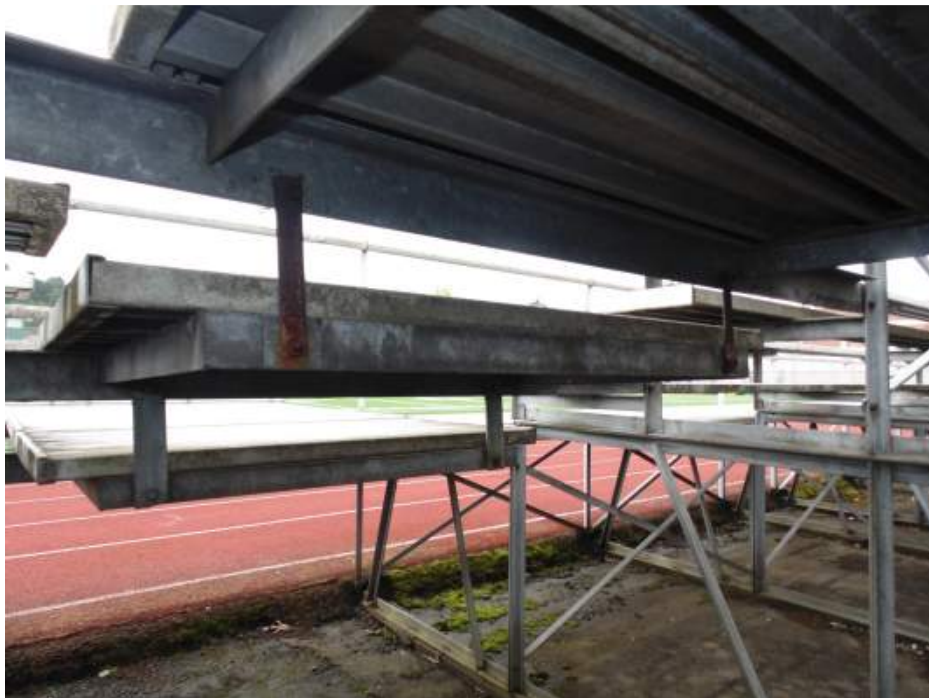
FIGURE S7: RUSTED PLATES AT STAIRS
