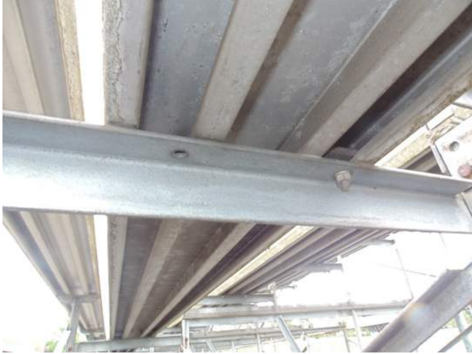
FIGURE B1: BOLT MISSING FOR SEAT/TREAD CONNECTION
