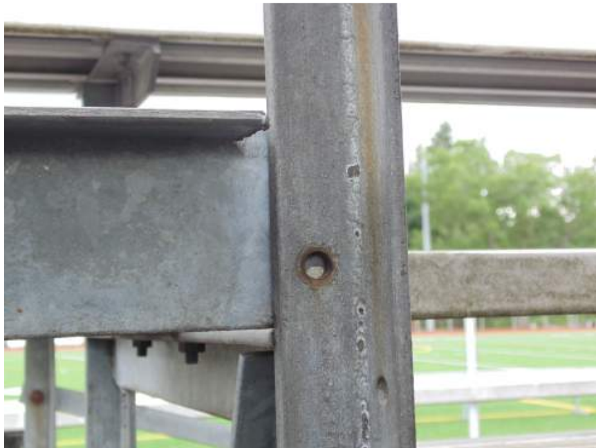
FIGURE B4: BOLT MISSING FOR STAIR ANGLE CONNECTION
