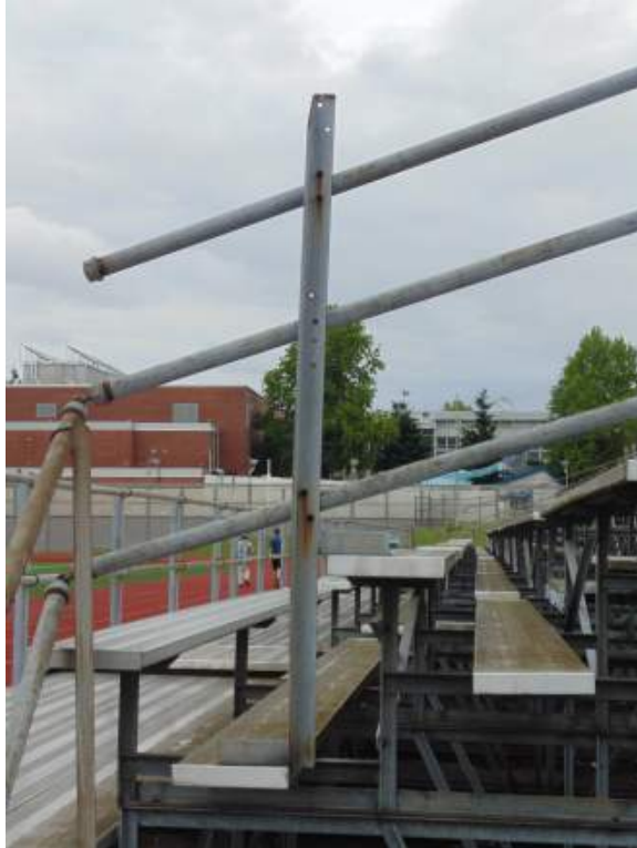
FIGURE B5: U-BOLT MISSING FOR RAILING CONNECTION
