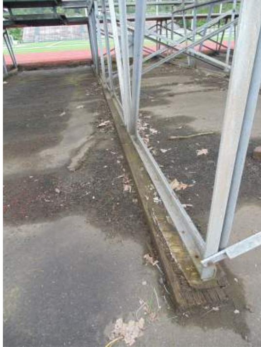
FIGURE W1: SUPPORTING WOOD MEMBER DETERIORATING
