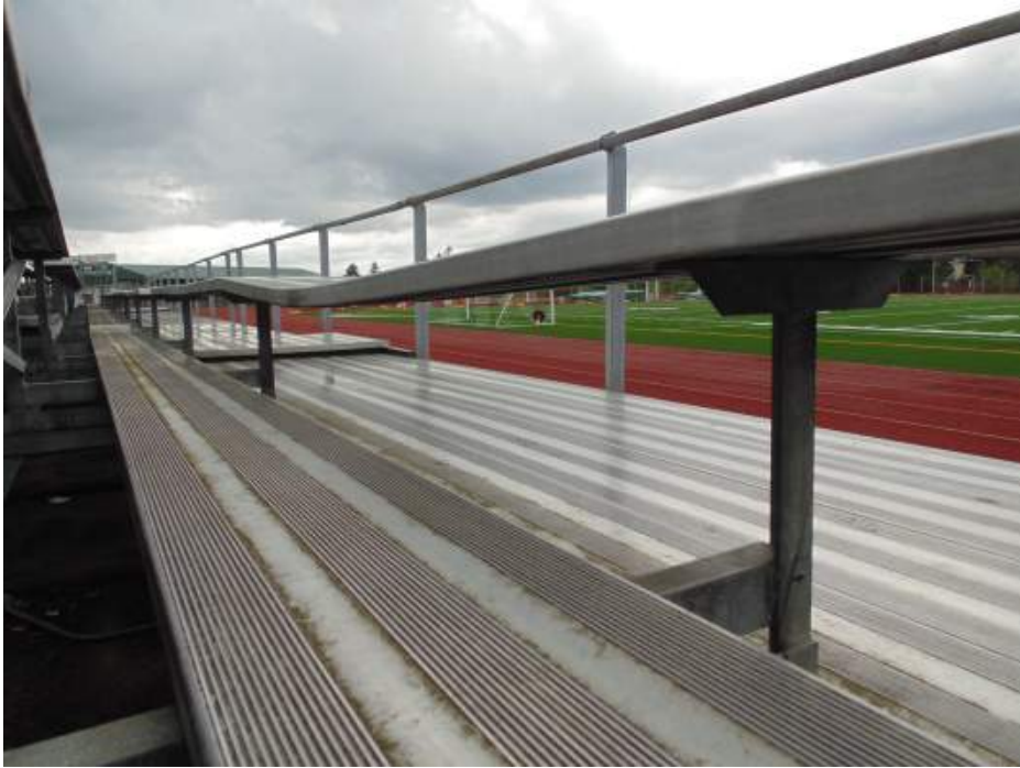
FIGURE S8: DAMAGED SEAT
