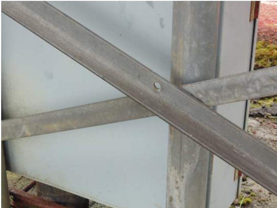
FIGURE B2: BOLT MISSING FOR BRACE CONNECTION
