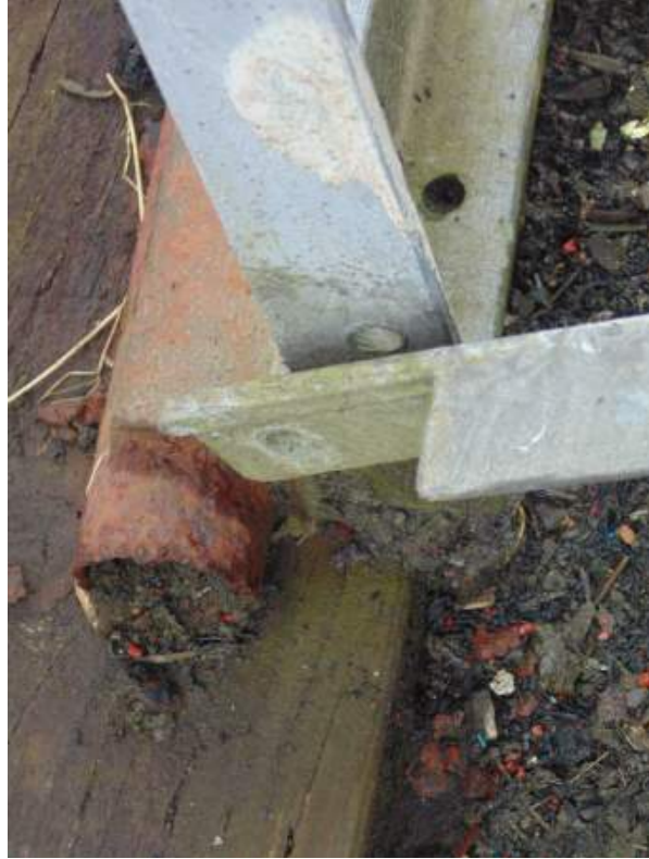
FIGURE B3: BOLT MISSING FOR FRAME TO FRAME CONNECTION
